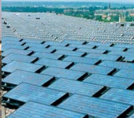
PV-Anlage Felix Platter-Spital | Basel ADEV Solarstrom AG 40 kWel | 1999
